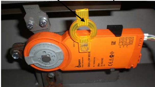
Instructions mode during a power failure
